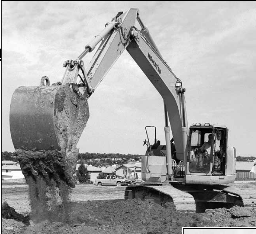
Larry Roloff uses a Komatsu PC228 “short-tail-swing” excavator on a recent site-development project in west Omaha.
